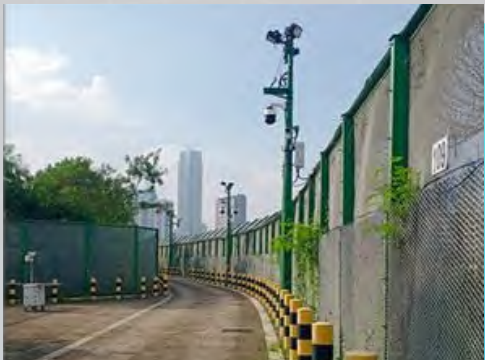
AI Fencing System, Lo Wu
